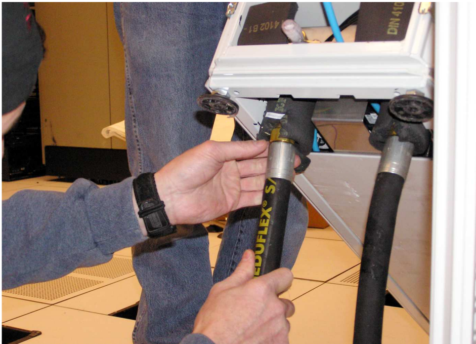
Supply & Return Connections
