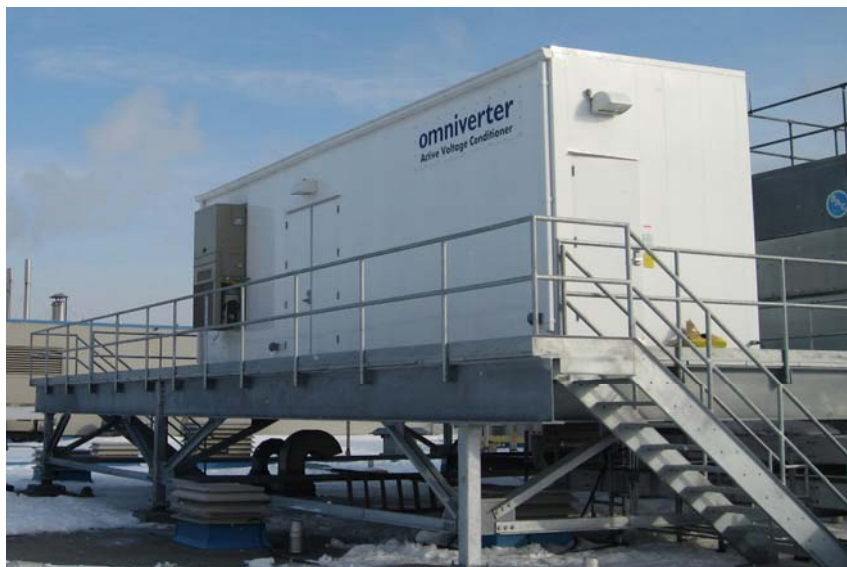
AVC Installed on the roof at Apotex
